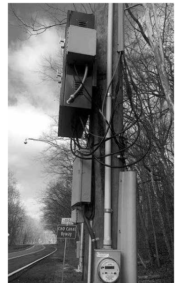
Small cellular base station equipment clutters a utility pole on MacArthur Blvd. in Potomac.
